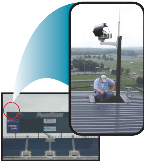
The PV16W was used for the scoreboards. A hole was cut into the roof and the poles were mounted to the internal skeleton.
